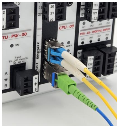
Figure 47 – 1 Double Optical Fiber + 1 Bidirectional Optical Fiber PA1187+PA1170B
