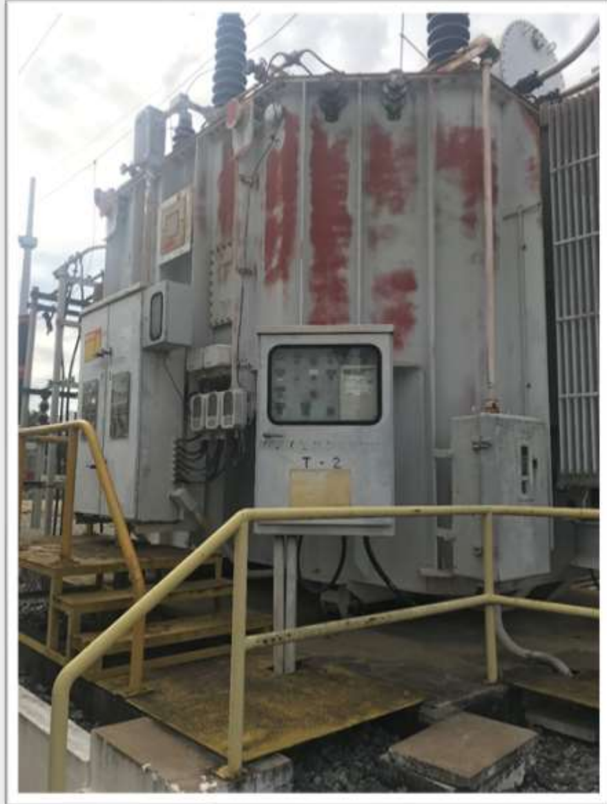
Power Transformer TUSA 138/88/13.8 Kv-20Mva
